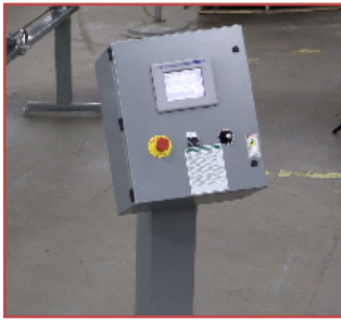
Free-Standing Allen-Bradley PanelView touch-screen controls
